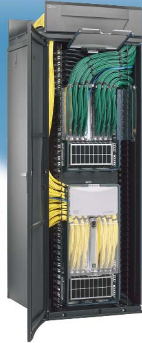
NET-ACCESS™ Cabinet managing two Cisco Nexus* 7010 switches
