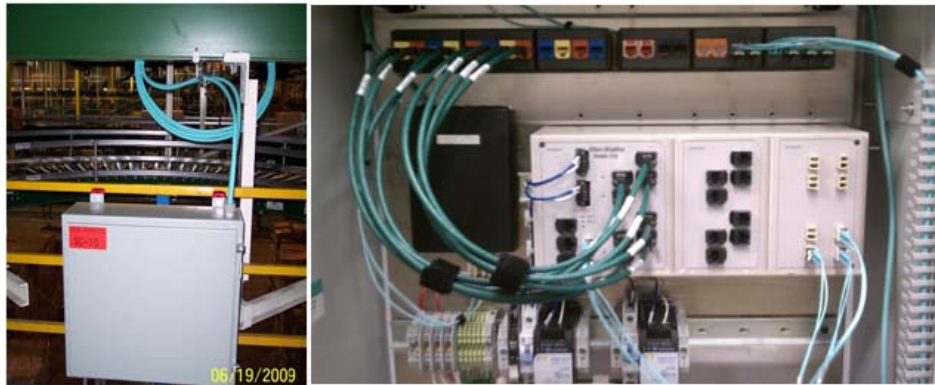
Figure 11 Sample Network Zone Fiber Optic Deployment
