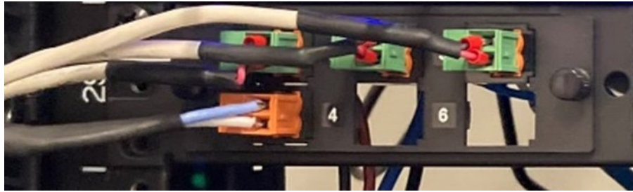
Connector Assembly in Patch Panel
